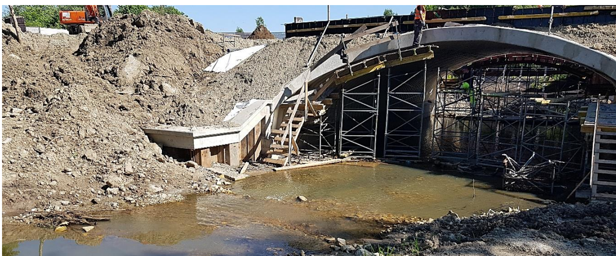
Figure 4. Reconstruction of a bridge over a creek along the DK state road. Source: SRK S.A. internal materials.
