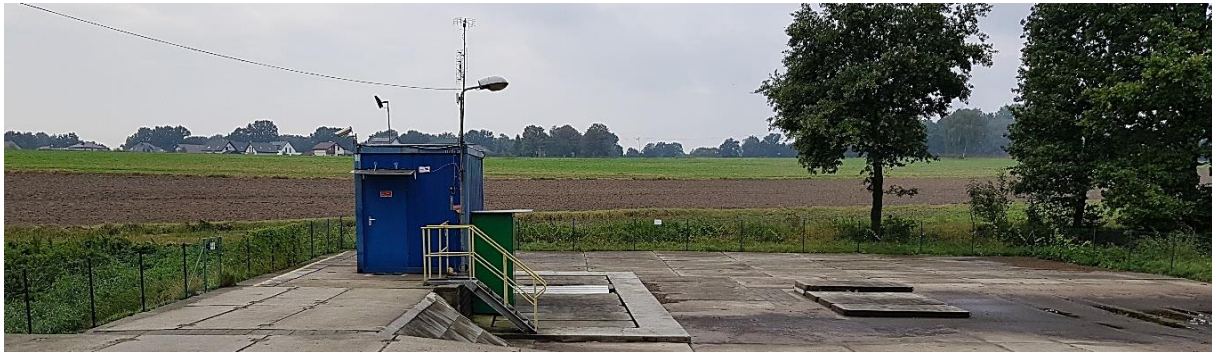
Figure 6. Equipment of the pumping station (view in SW direction).
