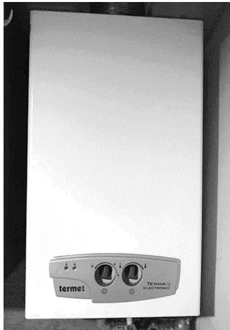
Figure 4. Tested gas-fired heater in an enclosure.
